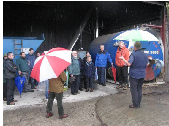
Figure 8: Farmstore big bale boiler installed in 1999 running on straw or waste wood loaded through the front door, beside a smaller boiler loaded with chips or pellets by a screw auger. (Photo: P. Burgess).
